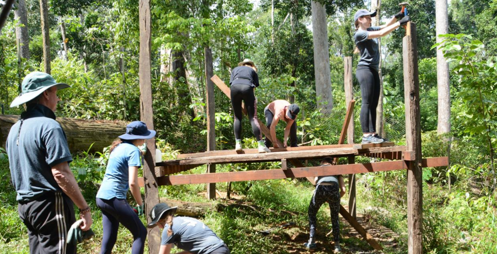
BATs group from the Diocesan School for Girls South Africa building a sun bear climbing structure in Pen D.
