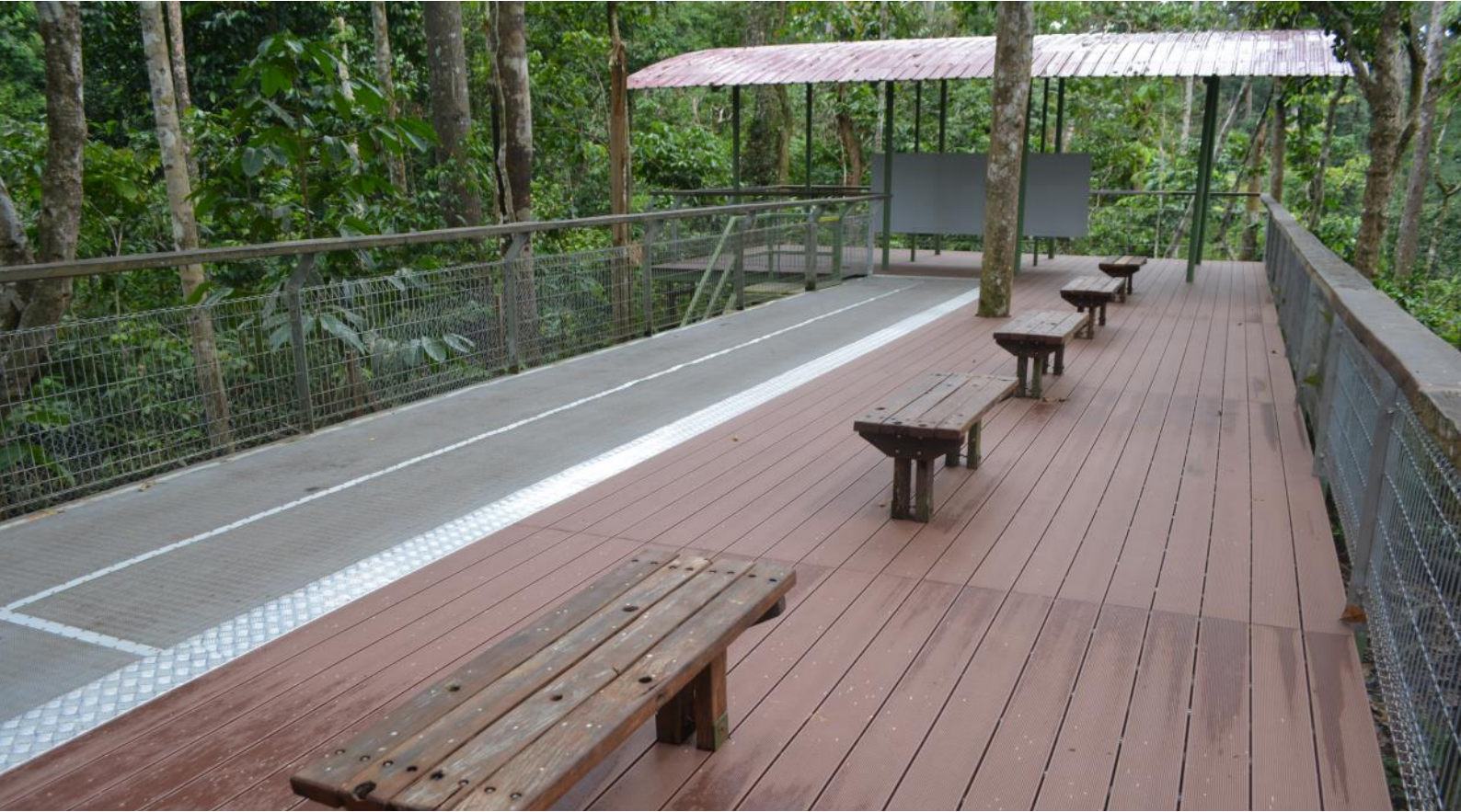
Top: Newly completed 2 nd Observation Platform. Bottom: 2 nd Observation Platform damaged by fallen trees.
