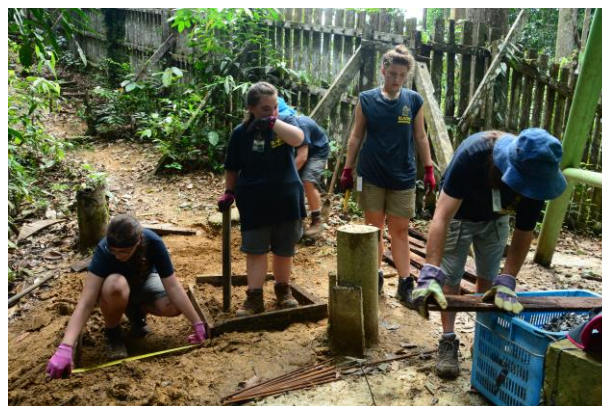
St Mary DSG Pretoria Team 1 repairing the perimeter walkways around the forest enclosure.
