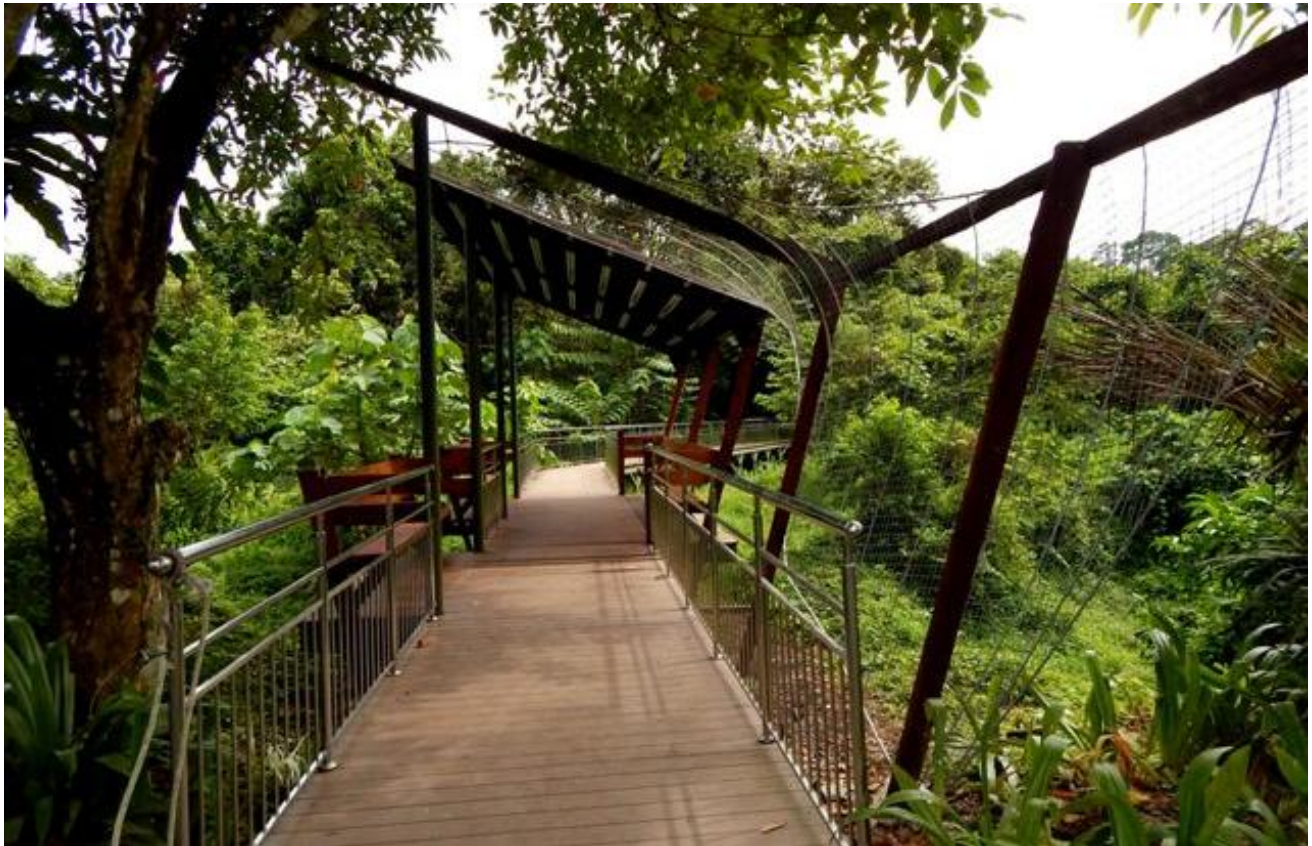
Newly constructed entrance gateway at the start of the access boardwalk to the visitor centre at BSBCC.
