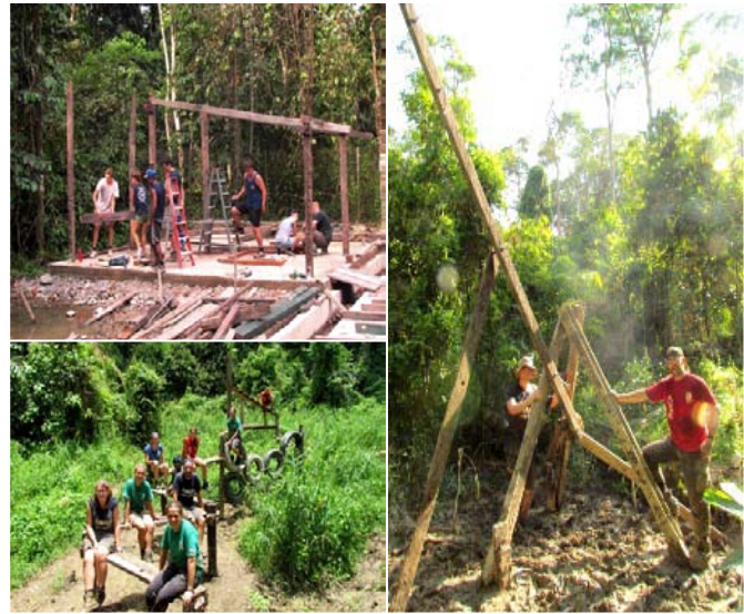
Top: Camps International volunteers building the foundation for the composting area. Bottom: Raleigh International volunteers with the completed bear climbing structure Right: Raleigh International volunteers and the foundation of the bear climbing structure.
