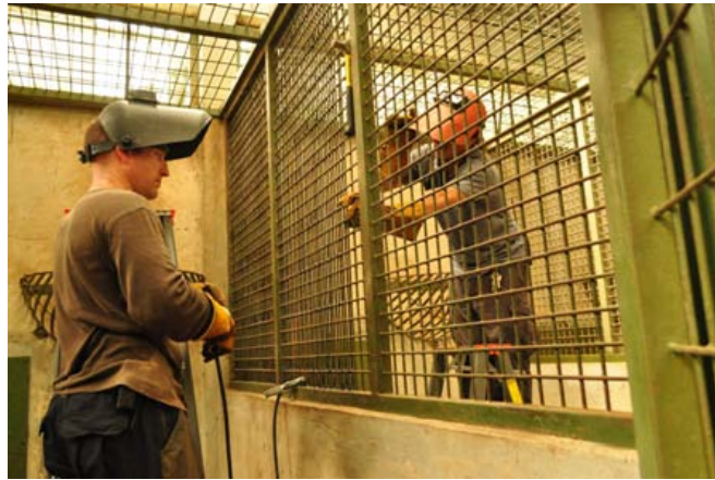
Special thanks to individual volunteer, Mr. Matthew Ford, for voluntarily leading the welding job together with contractors and our general workers.
