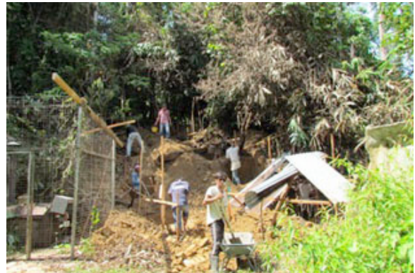
Work starting on one of the trails leading to the observation platform from the old bear house.
