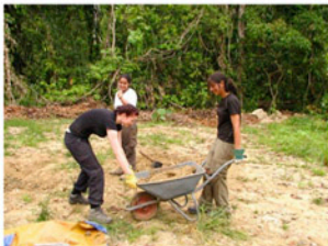
Wilderness Expertise volunteers collecting soil to level the ground under the new bear house.
